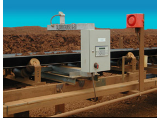
MA-500 Installation on NICKEL ORE
