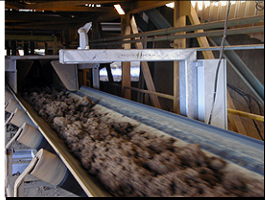
MA-500 Installation at SLN – New Caledonia
