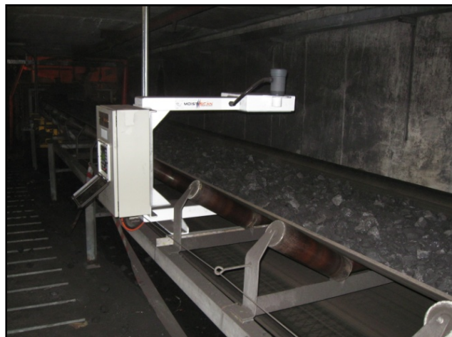
MA-500HD installed on conveyor to measure the moisture in coal entering site
