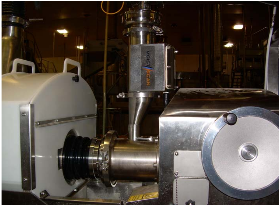
Moistscan located above extruder, hydrator is located above MoistScan ® ( off picture)
