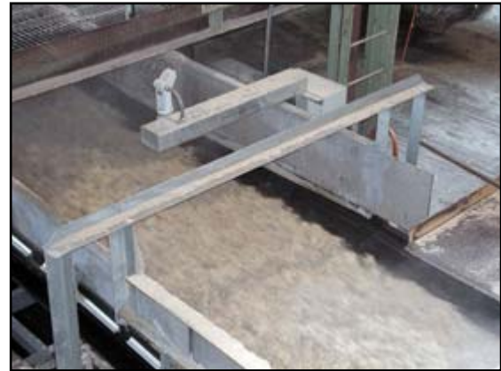
MA-500 installed on conveyor measuring the moisture in bagasse
